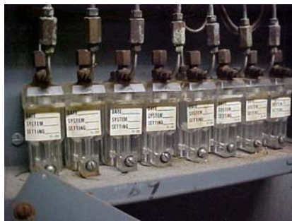
Elemental Mercury Fire Alarm System
