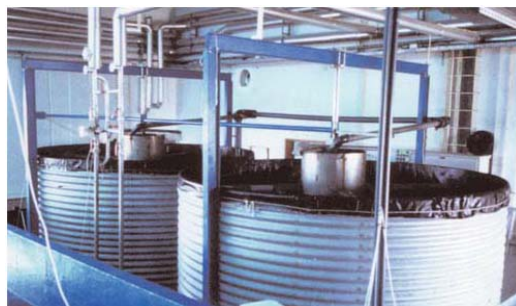
Trickling Filter in a WWT Plant; Photo Source: Food & Agriculture Organization (FAO)
